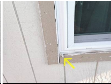
Cracking of trim
