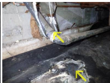
Leak and puddle
