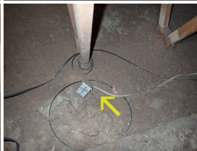
Secure wire and junction box
